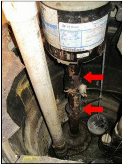
24. Rusted sump pump pipe.
