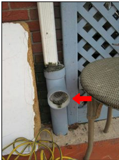
10. Open pipe at back downspout drain.
