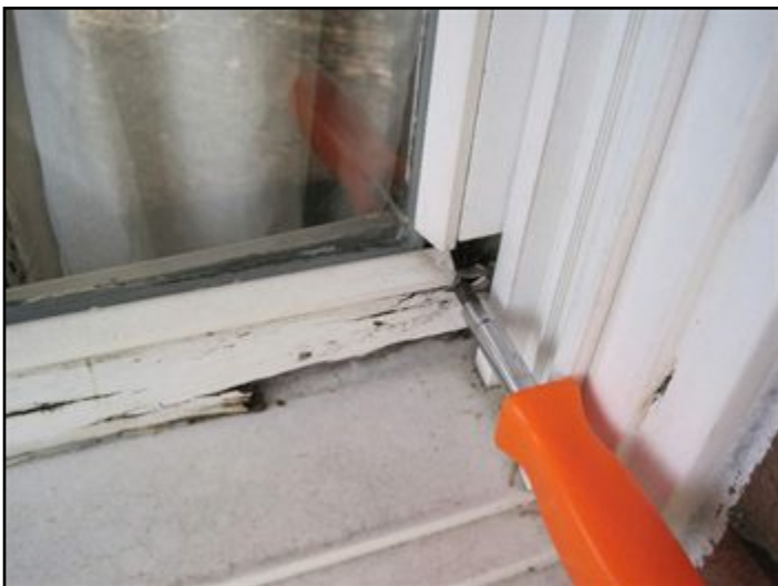
26. Rotted window (living room window).
