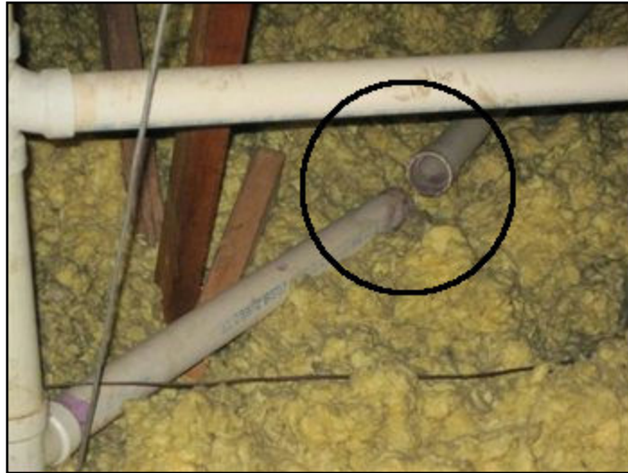
23. Disconnected plumbing vent pipe in attic.
