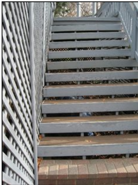
15. Loose/tipped stairs at deck.
