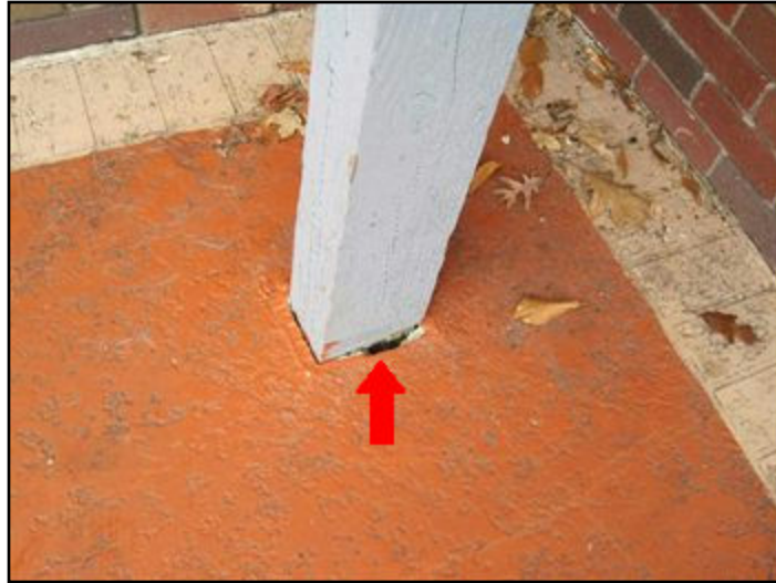
14. Rot progress at deck posts.
