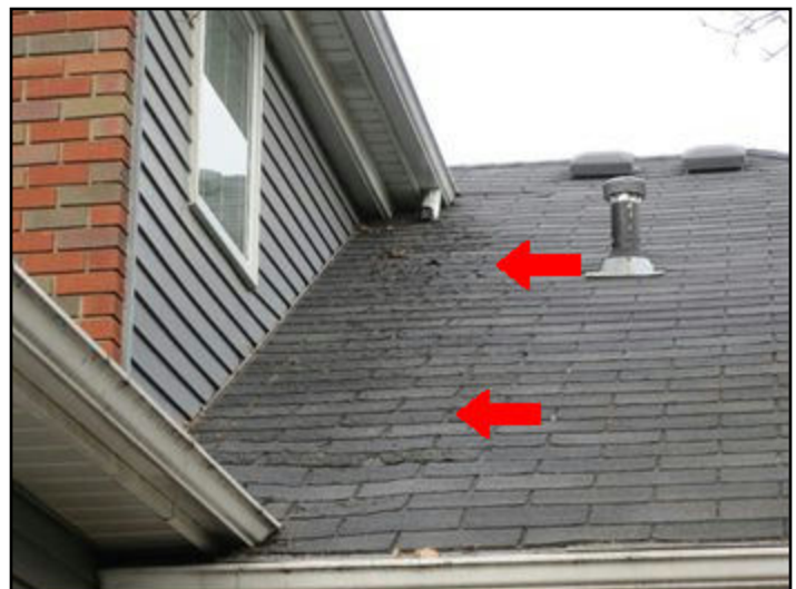
2. Area of significantly worn shingles.
