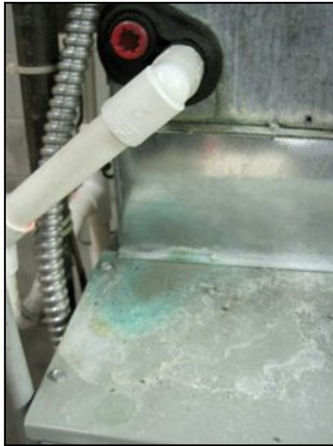
21. Condensate leak evident at furnace.
