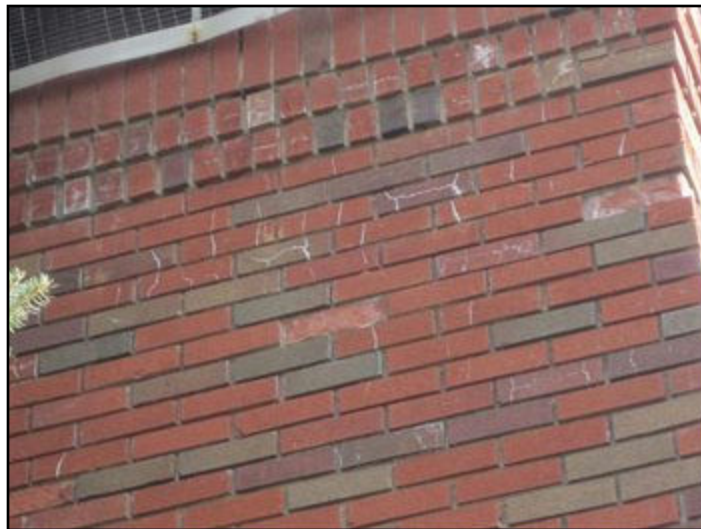
13. Cracked/spalled brick at chimney top.
