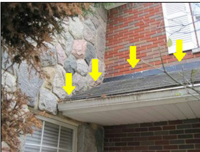
1. Flashing/caulking needed at re-roof.
