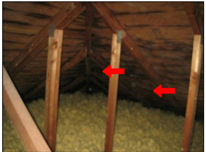
6. Mold on roof sheathing (NW corner of attic).
