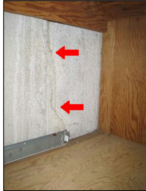
29. Leak stains at foundation crack.
