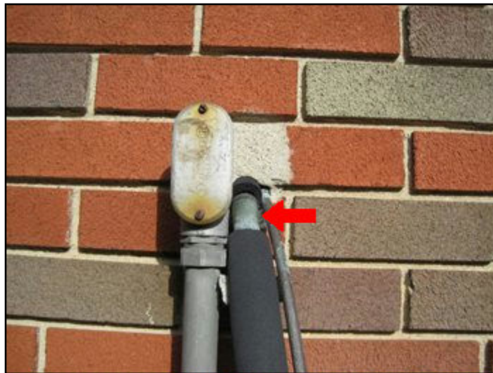
22. Insulation missing for refrigerant lines-back
