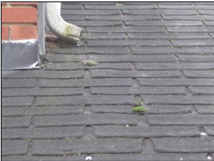
5. Worn shingles (example location).
