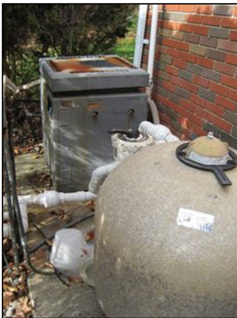
7. Old pool filter/heater/pump system.
