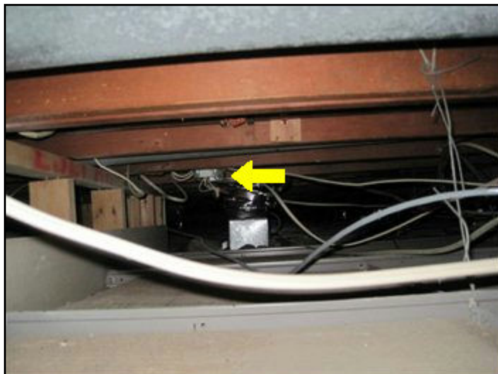
20. Open junction box, loose wire above ceiling.
