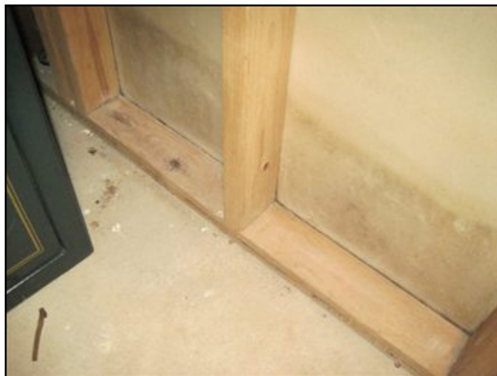
25. Mold on drywall in basement, at water meter..
