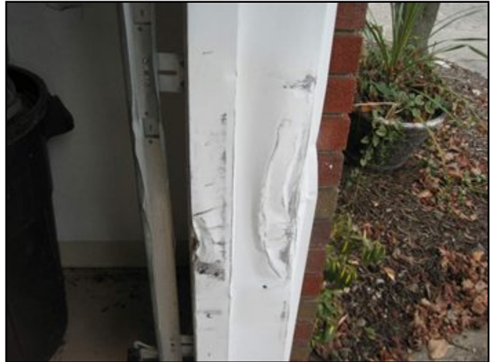
9. Damaged trim at garage door opening.
