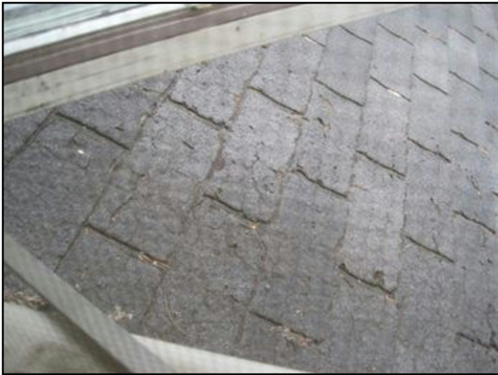
3. Significant shingle damage (example).
