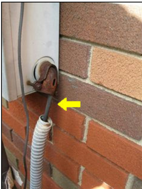
19. Open conduit at AC subpanel in back.
