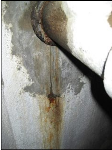
28. Active leak at main drain near water meter.
