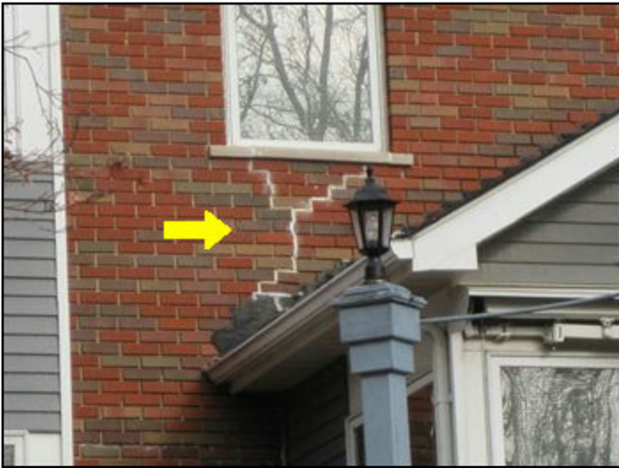
11. Area of cracks at brick joints in back.
